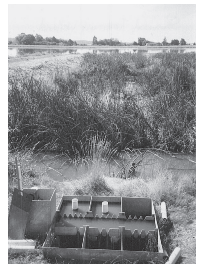
After undergoing primary treatment in a partially aerated pond, wastewater flows to a “splitter box” with V-notches that control the loading rates into four wetland cells.
